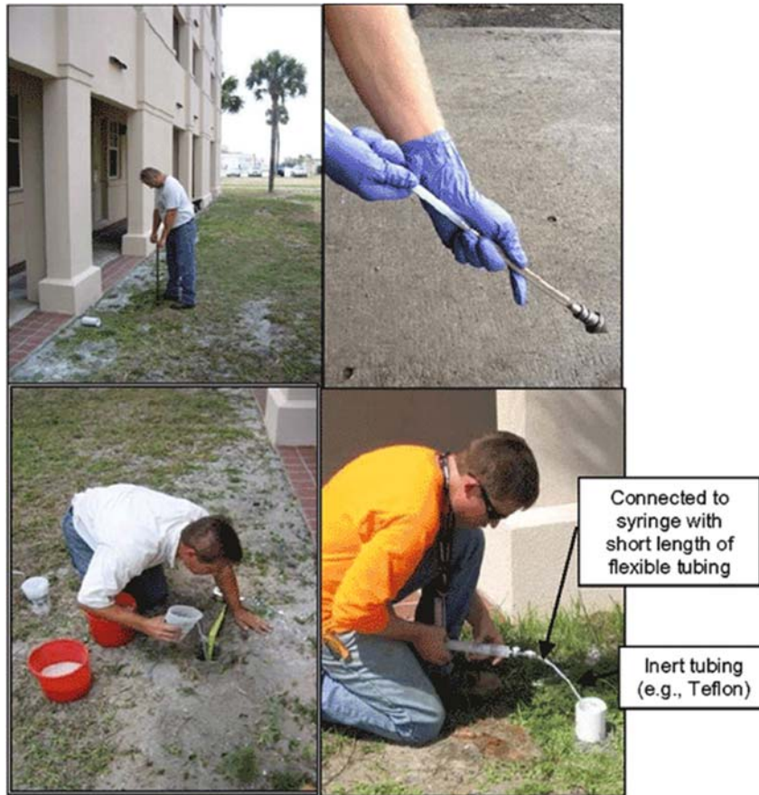
Figure 7-26 Installation of a Permanent Soil Vapor Probe. Upper left photo: Hand augering the borehole. Upper right photo: Preparation of soil vapor sampling point. Bottom left photo: Hydrating the bentonite seal. Tape used to measure depth of borehole, sand pack, and bentonite. Bottom right photo: Purging the completed vapor probe. Surface completion is a 9-inch length of 3-inch diameter Schedule 40 PVC pipe placed into upper 6 inches of the borehole around the probe tubing. A slip cap is placed over the PVC when not purging/sampling.
