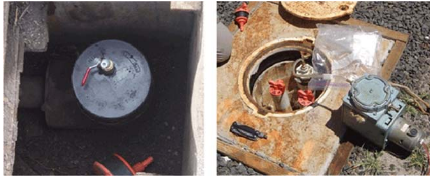
Figure 7-24 Vapor Point Completions Left: Surface completion of flush-mounted well with valve installed. Right: Flush mounted nested well with Swagelok fittings; well in background being purged using an electric pump set at a draw rate of 200 ml/minute.
