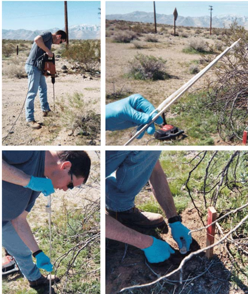
Figure 7-41: Installing a (Qualitative) Passive Soil Vapor Sample Collector by Hand. The hole is drilled using a roto-hammer. The soil vapor sample collector is installed using an insertion rod. The hole is then covered.
