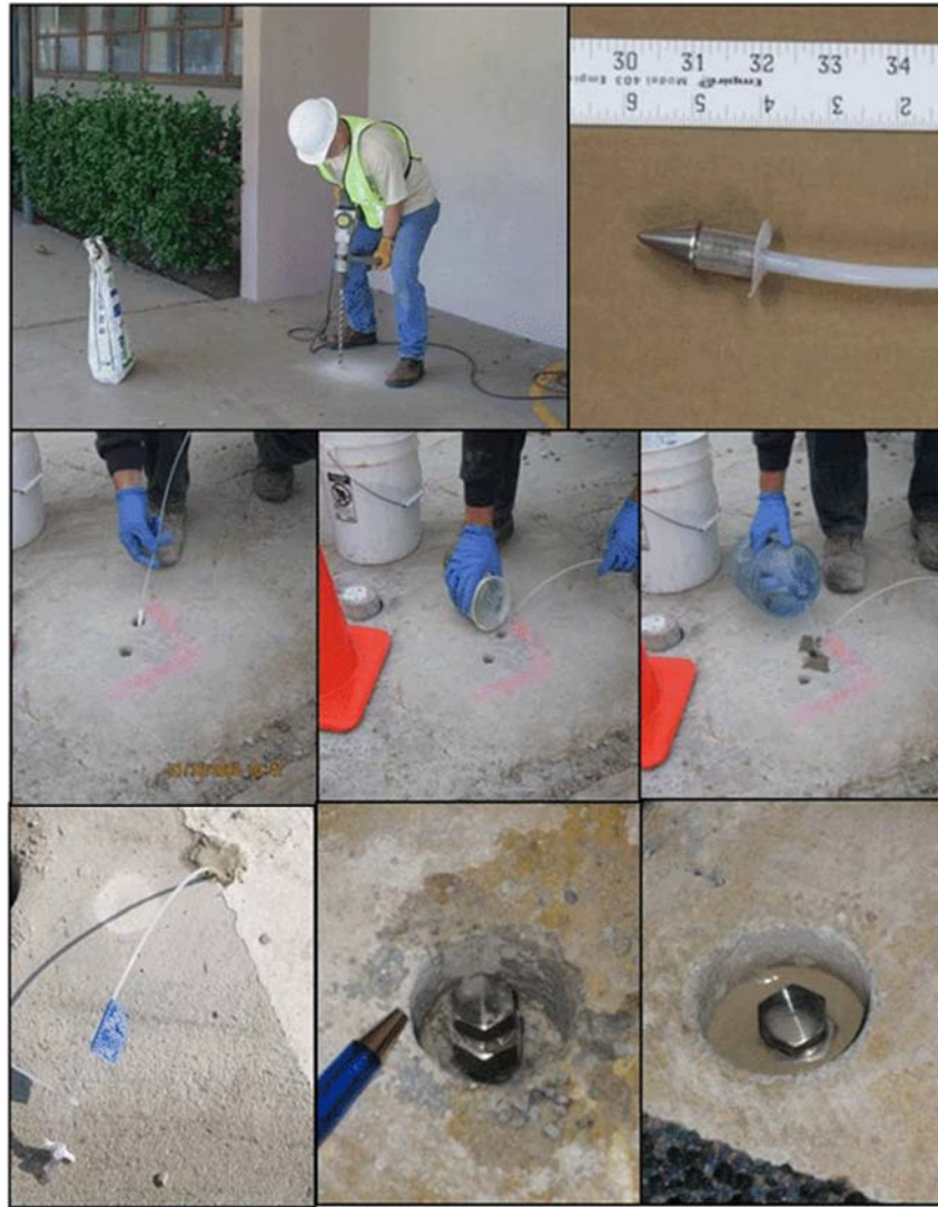
Figure 7-28 Sub-Slab Soil Vapor Sampling Probes Upper left photo: Drilling hole with hand-held rotary hammer drill. Upper right photo: Temporary probe tip. Middle sequence: Inserting probe assembly into hole, pouring granular bentonite, hydrating bentonite seal. Bottom Left: Temporary probe completion. Bottom Middle and Right: Vapor probe with Swagelok termination fitted to hole (note larger diameter hole near surface), final completion with Swagelok fitting on tubing cemented in place (see Figure 7-25 ).
