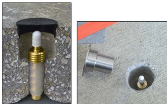
Figure 7-30: Installation of a Vapor Pin™ with a silicon sleeve directly into slab for collection of subslab vapor samples (screw-on protective cap shown in photo to right). Sample collection tubing is connected directly to the top of the probe point (after rubber slip-on cap is removed) and the sample drawn through the base.
